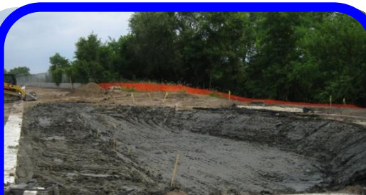
The cells were over-excavated and clay lined to prevent side hill seepage to bluff
